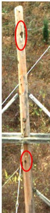
STR. 429-6 - Woodpecker Holes - Vertical Pole Cracking at Woodpecker Holes
